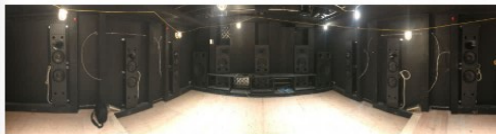
A photo illustrating the system in place prior to acoustics and finishes. Photo Credit: Robert Bracero, Roberts Home Audio & Video, Inc.
